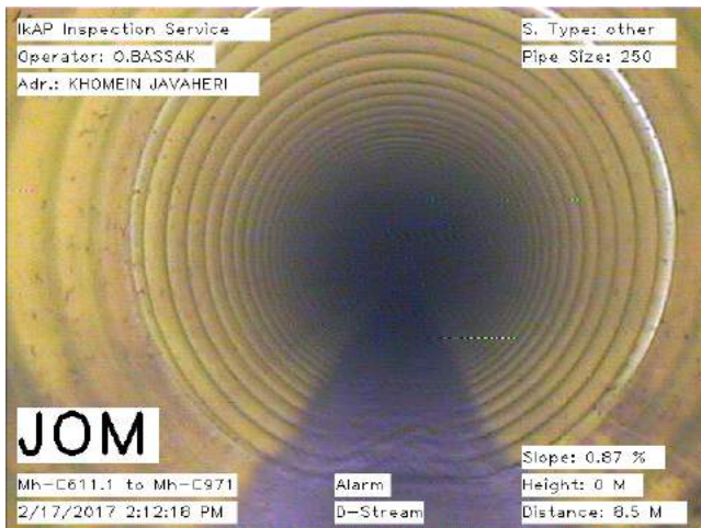
Photo : 2.jpg 8.5 m, Joint Offset Medium # 3
