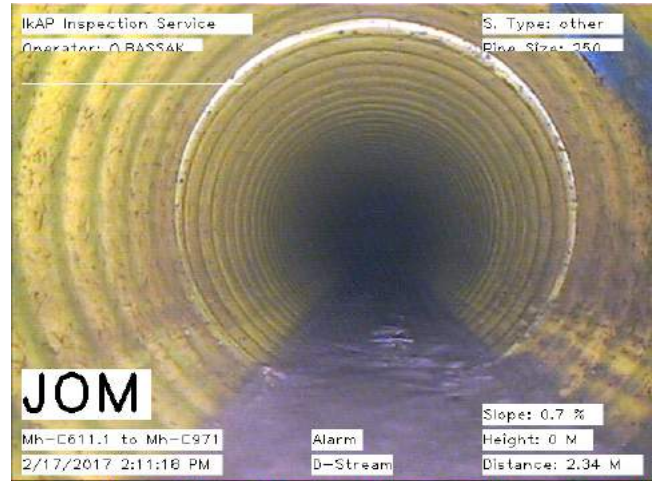
Photo : 1.jpg 2.34 m, Joint Offset Medium # 2
