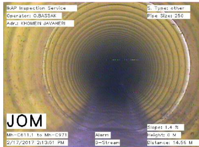
Photo : 3.jpg 14.56 m, Joint Offset Medium # 4
